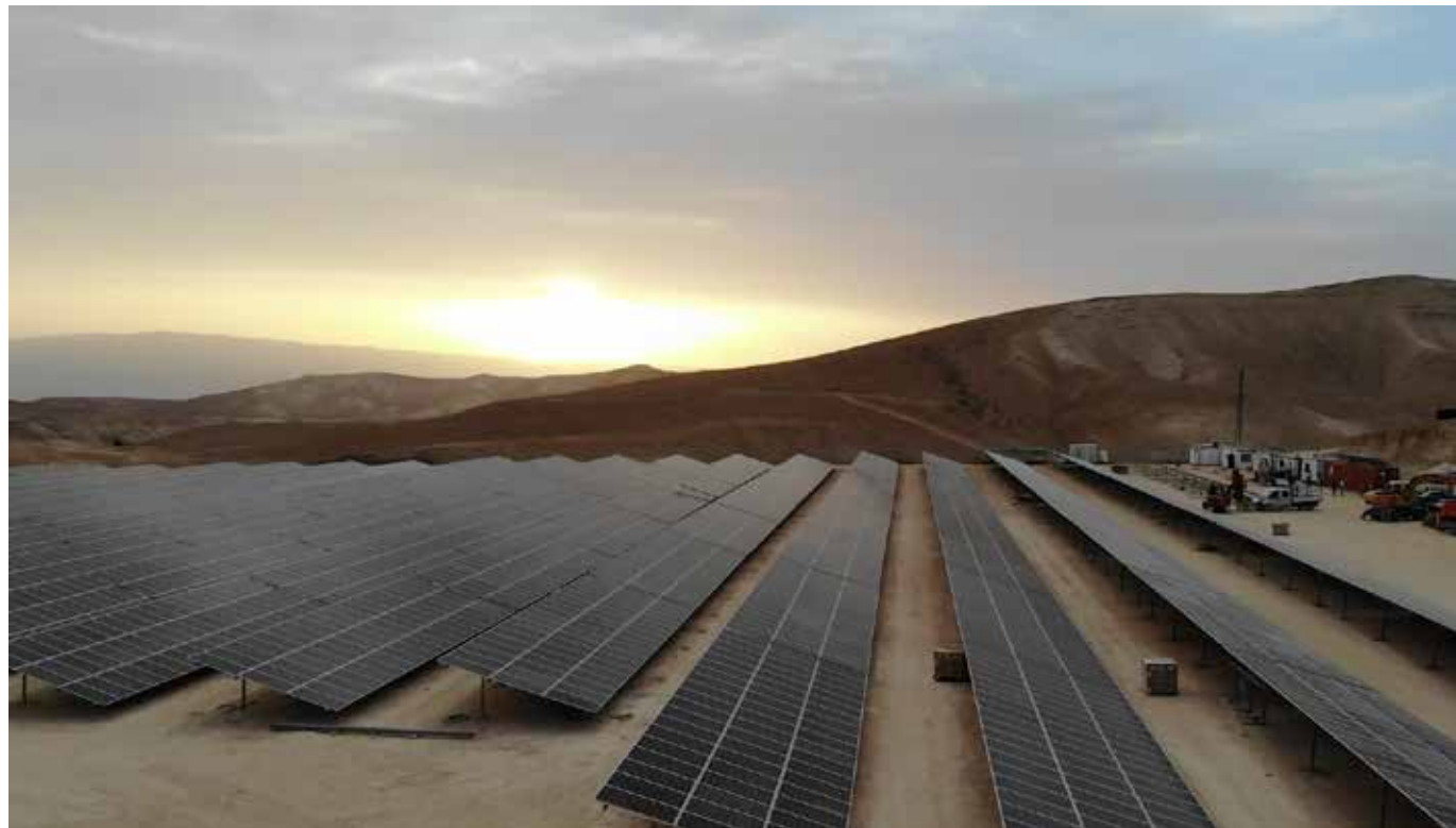
Initial installation activities of the "Noor Jericho" solar park, where TNB has a stake of 1,127 Mw.
