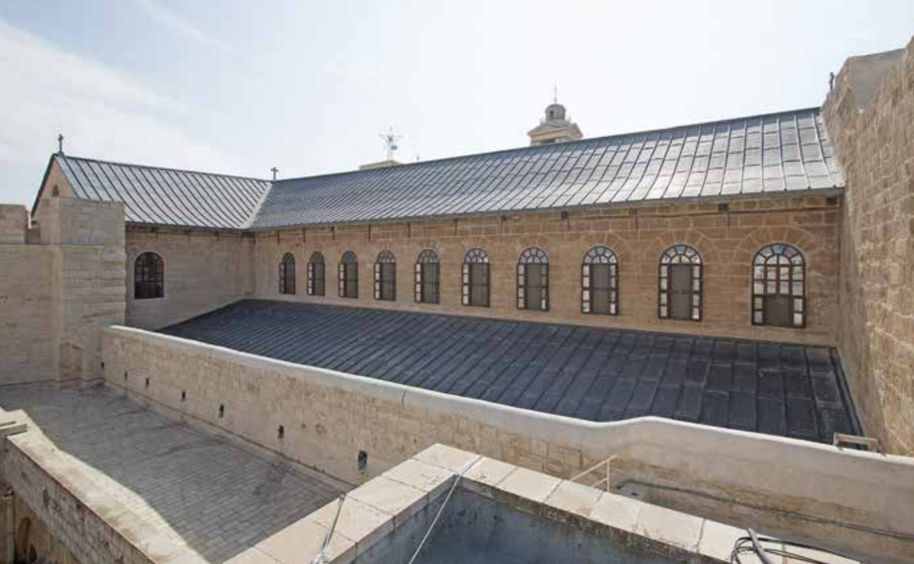
The north nave of the basilica and the lead roof after the restorative works.
