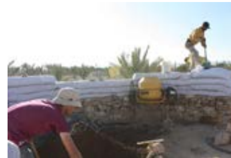
Moon Cocoon under construction, Jericho. Designer Shams Ard Design Studio. Photo courtesy of Shams Ard.
