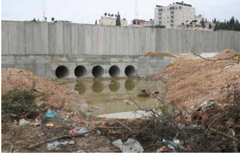
A usual sight when a waste water network is blocked.
