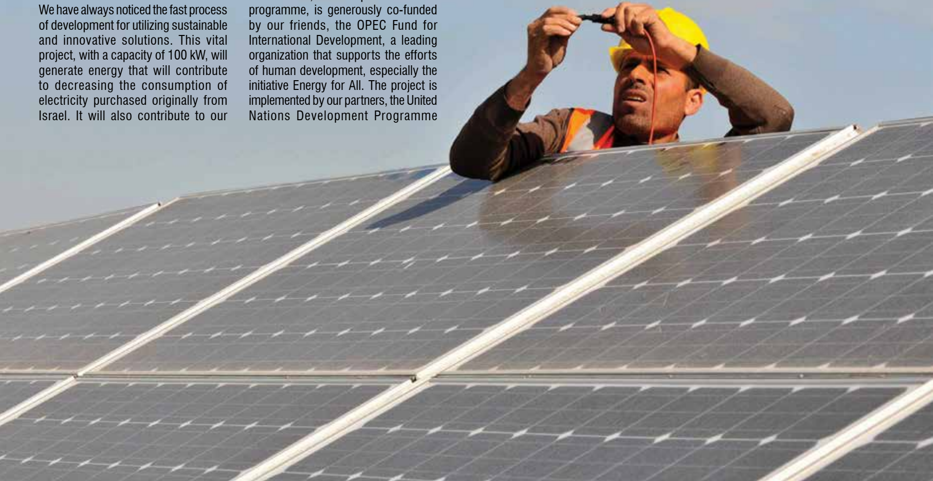
After installation, a worker connecting the solar panels for energy generation. Photo by Shareef Sarhan - ©UNDP/PAPP.
