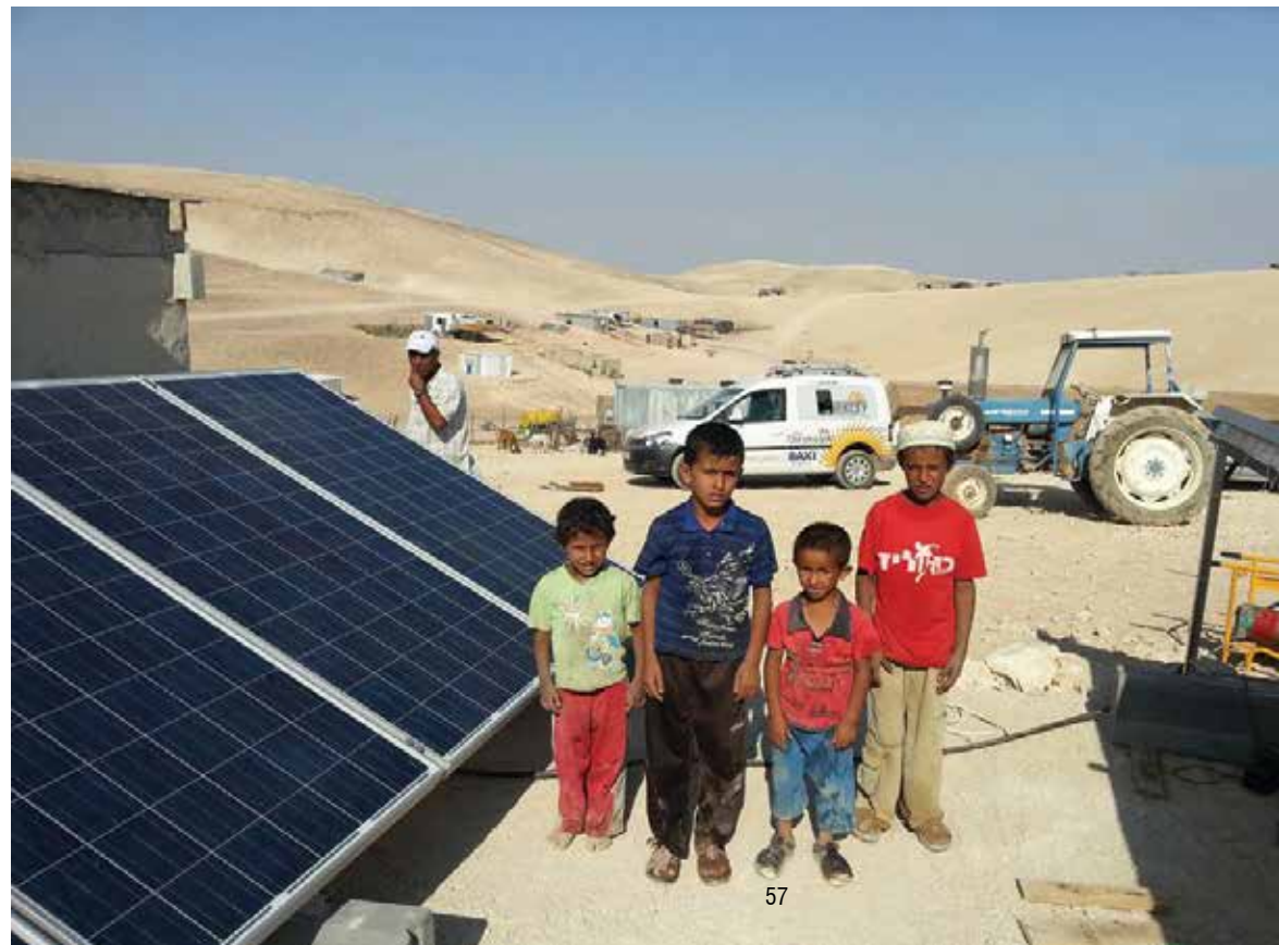
Off-grid solar PV system for thirty bedouin families at Al-Rawaeen community, near Hebron.
