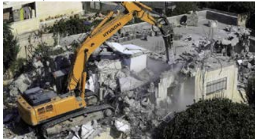
A house in northern Jerusalem being demolished because it lacks the necessary construction permit. According to the Israeli land-planning and zoning system, 87 percent of Jerusalem is off-limits to Palestinians, forcing them to build without proper construction permits.
