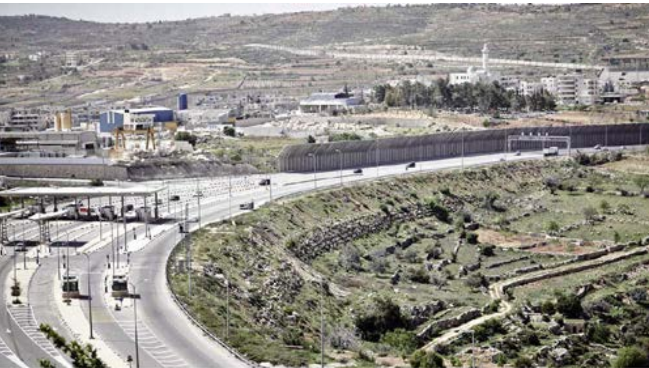
A section of the 4.35-kilometer-long wall being built by Israel on the lands of Al-Khader. Once completed, it will separate the town of Al-Khader from 68 percent of its lands and properties. The Israeli military checkpoint that can be seen on the left was constructed on the lands of Al-Khader. No Palestinian residents of Al-Khader are allowed to pass through this checkpoint, even if they obtained a military permit. ©Patrick Kruse/OPGAI.
